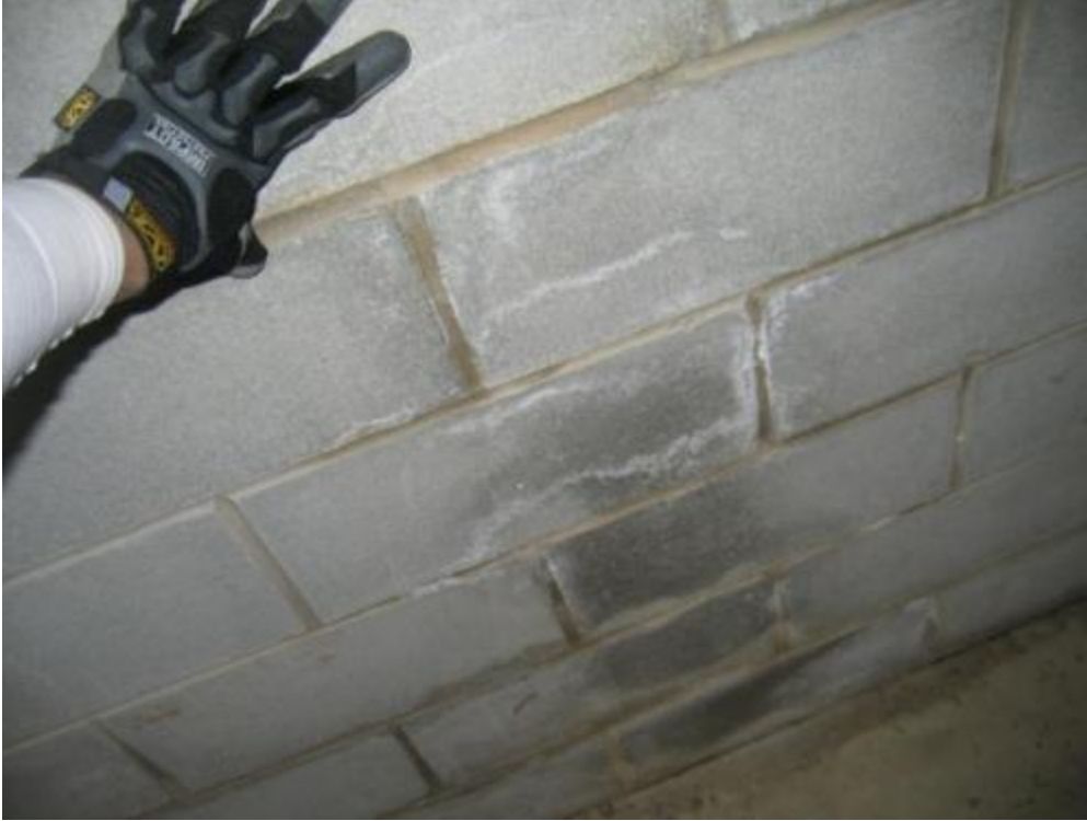
Efflorescence is indicated by the white deposits on the concrete block foundation wall, which is a result of moisture intrusion through the masonry.
