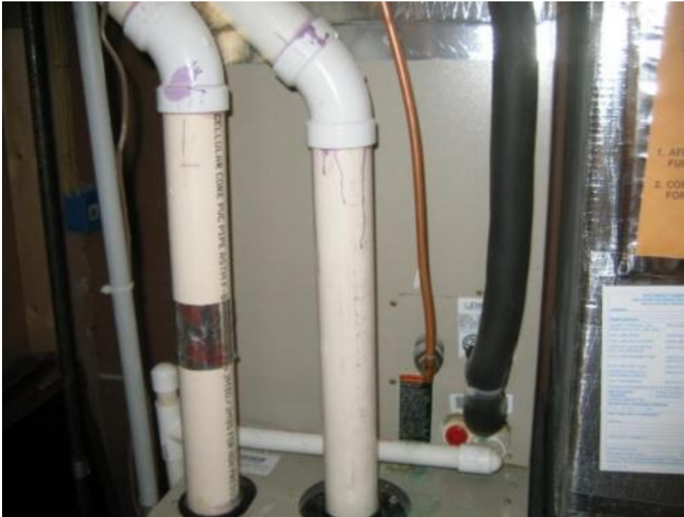
The inspection image above is of an evaporator coil unit installed on a high-efficiency, gas-fired, forced-air furnace.
