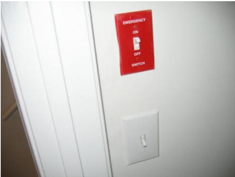
This is an inspection image of an emergency shutoff switch, a normal operating control.
