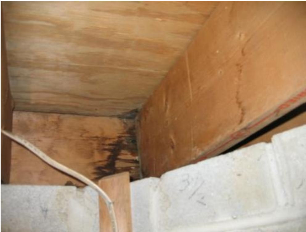
Indications of moisture intrusion was observed at the band/rim wooden joist located above the concrete block foundation wall. The water marks are an indication of the problem.
