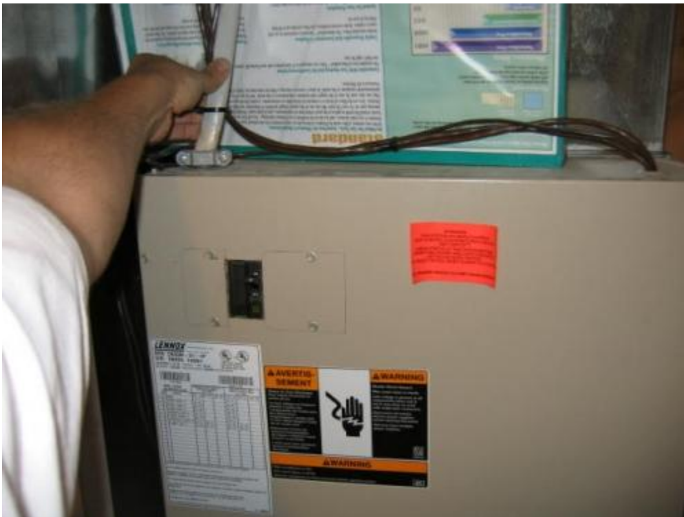
The inspection image above is of an electric heat pump furnace, and the inspector is touching the electrical line to the interior air handler unit.
