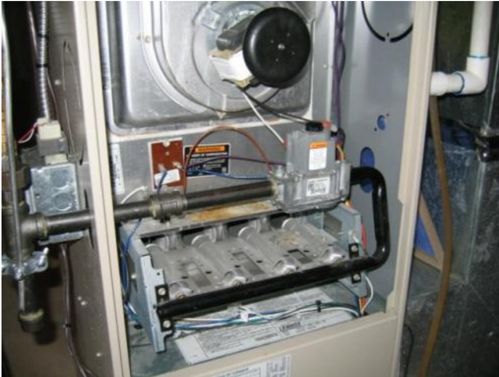
The inspection image above is a mid-efficiency, gas-fired, forced-air furnace.
