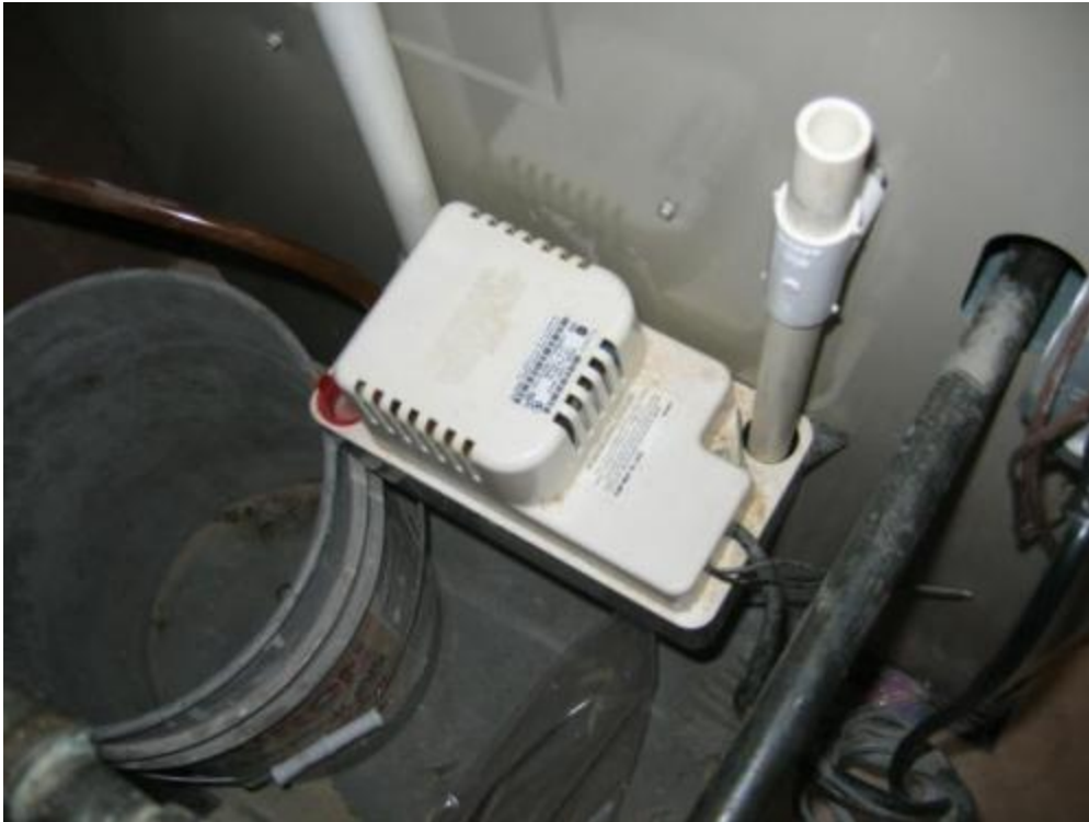
The condensate drains into a condensate pump resting next to the furnace.
