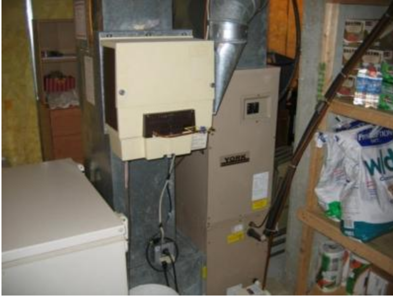
The image above is of a heat pump system.
