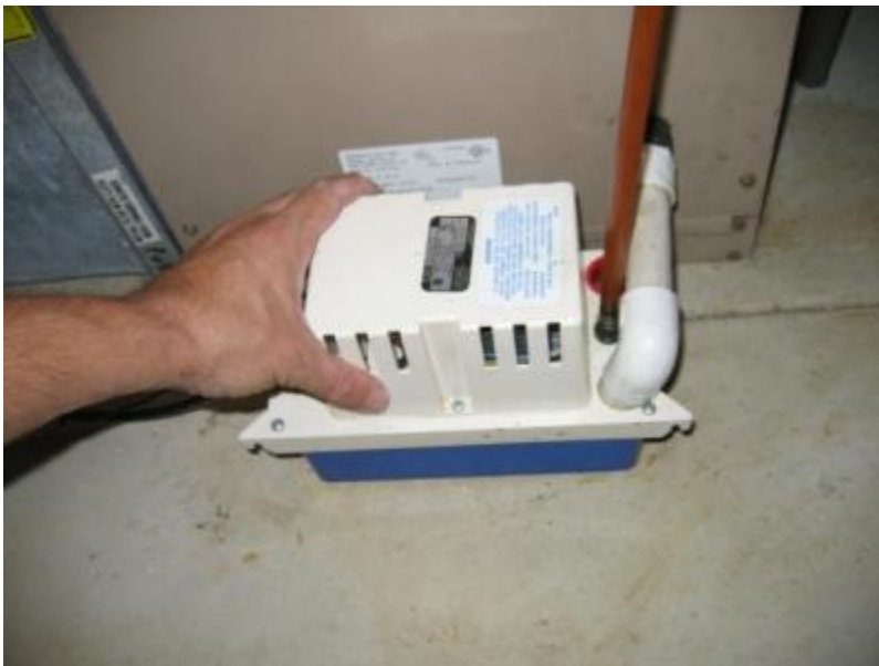
The image above is of a condensate pump, which is a component of the heat pump system. A System Is an Assembly
